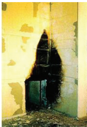
Figure 16: Damage of the test sample: PU insulation layer
