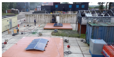
Figure 24: Arrangement of PV system on the roof assemblies
