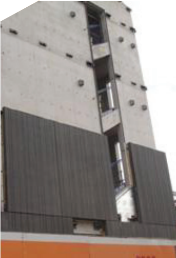
Figure 7: External cladding applied as soon as possible to insulated parts, stage by stage (Ventilated façade, Manchester, UK, August 2010)
